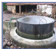
Rural Energy Systems
